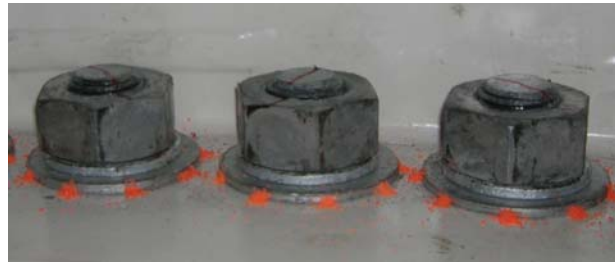
An M36 Euro Squirter installed in a wind turbine flange.
