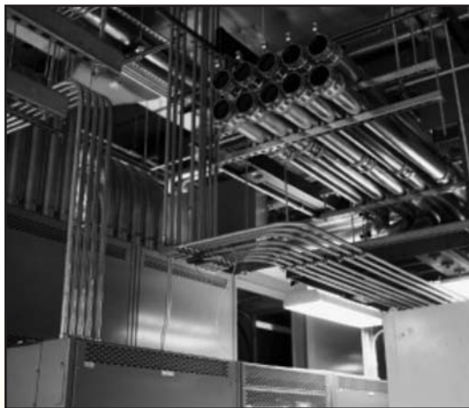
"Contractors Boost Productivity by Supporting Duct and Conduit with SOLNs"
