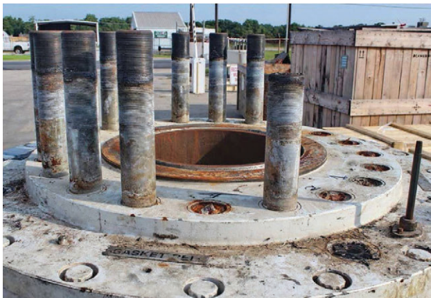
THIS PHOTO OF A SUBSEA OIL WELL COMPONENT WITH FAILED BOLTING APPEARED IN MANY REPORTS AND PUBLICATIONS, INCLUDING THE WALL STREET JOURNAL. THE STUDS ARE 3" IN DIAMETER.
